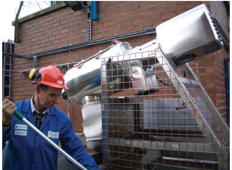
The Liquid Solid Separator in use at the Finlay's plant
