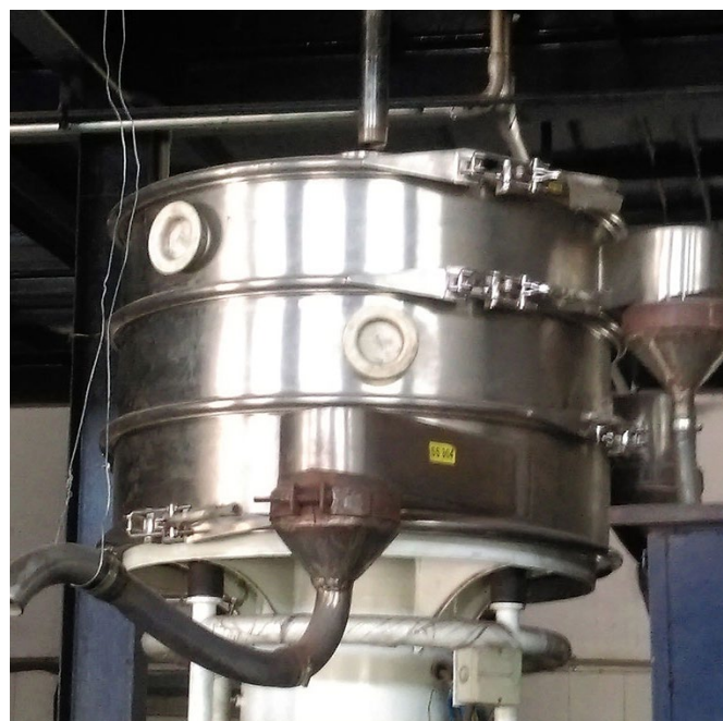
Figure 1. The Finex Ultima™ installed at Adishiv Forge Rajkot unit
