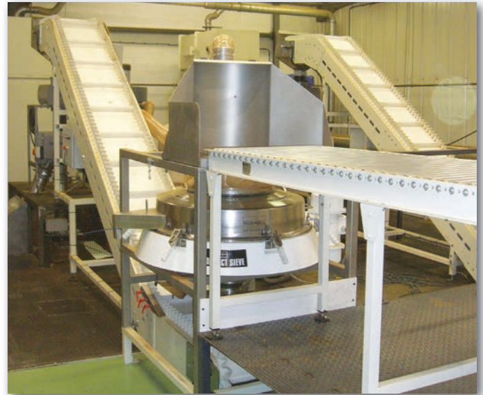
Figure 1. One of the Compact 3in1 Sieves™ installed at Clipper Teas
