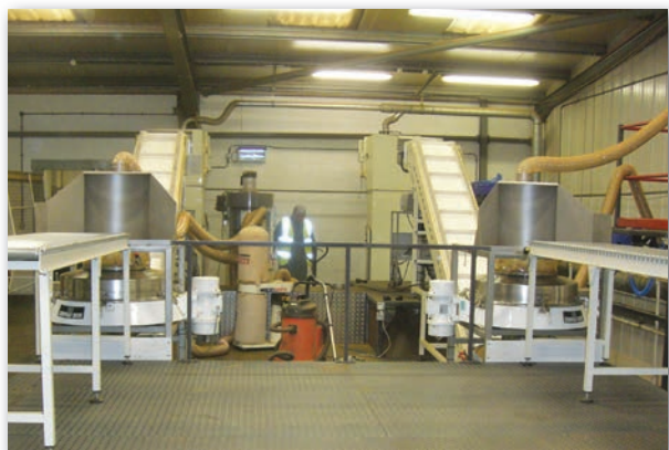
Figure 2. Two Compact 3in1 Sieves™ installed in two identical production lines
